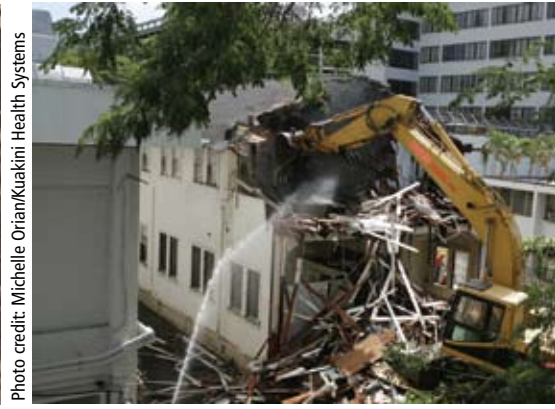
Tajiri Lumber handled the demolition of this structure at Kuakini Hospital in April 2009.
