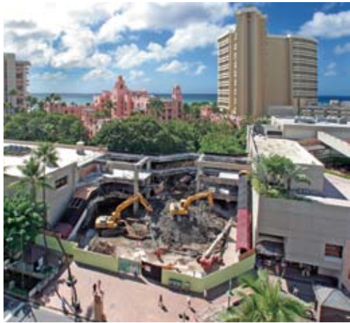
Nuprecon handled the demolition phase of the Royal Hawaiian Center's multimillion-dollar transformation project.
