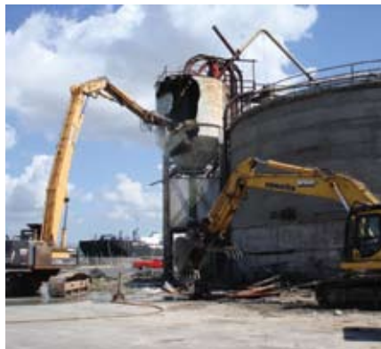
Northwest Demolition & Dismantling crews work with surgical precision to remove a tank at Sand Island.
