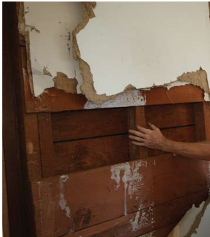
Right, Re-use Hawaii's Quinn Vittum marvels at the quantity of first-rate lumber his crew is about to recover from a 100-year-old, 4,000-square-foot home in Manoa.
