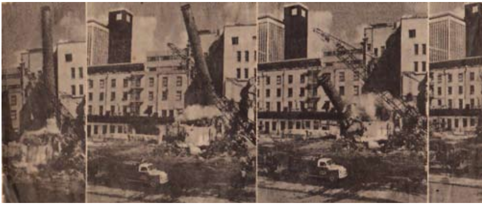
The chimney of the Alexander Young Hotel topples down in this frame-by-frame photo dated 1959. Tajiri Lumber was careful not to disturb a nearby live transformer vault, which if damaged, would knock out power all over Honolulu.
